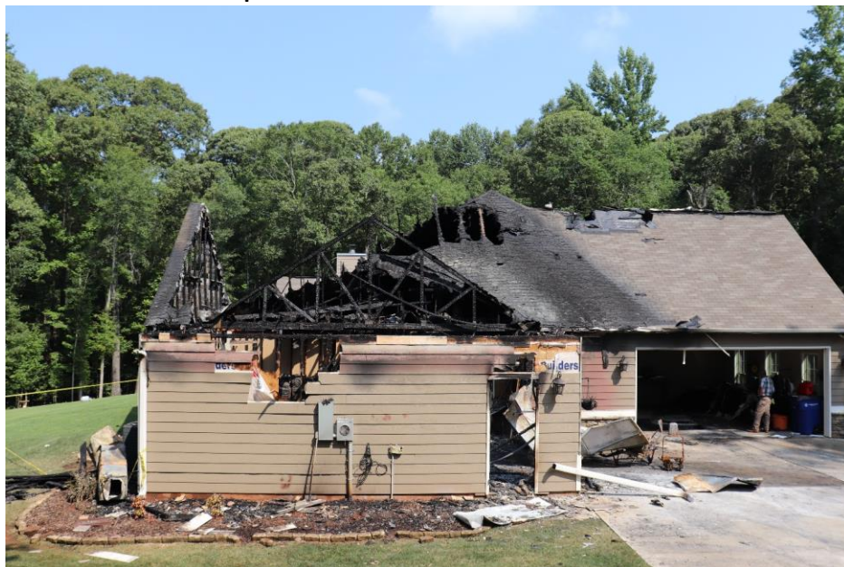
Structure fire at 2191 Mooty Bridge
