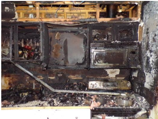
Structure Fire on Everette Street
